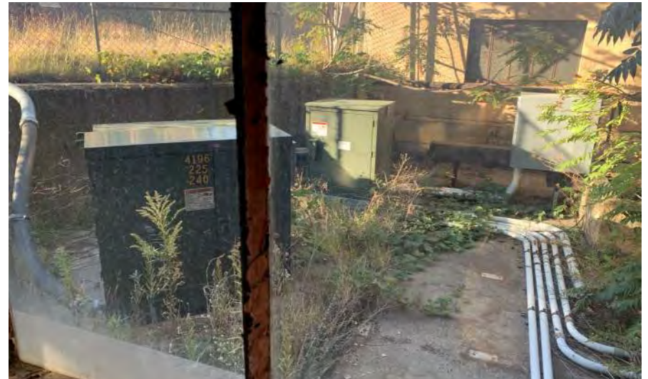
Electrical transformers outside south side of building
