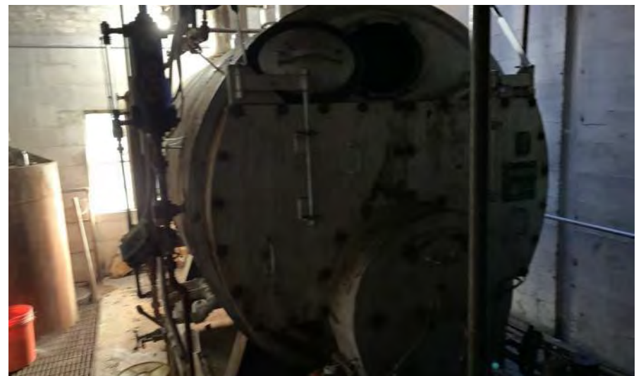
Boiler in boiler room
