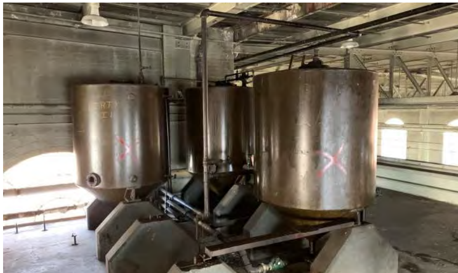
Empty dirty oil and new oil tanks on third floor mezzanine
