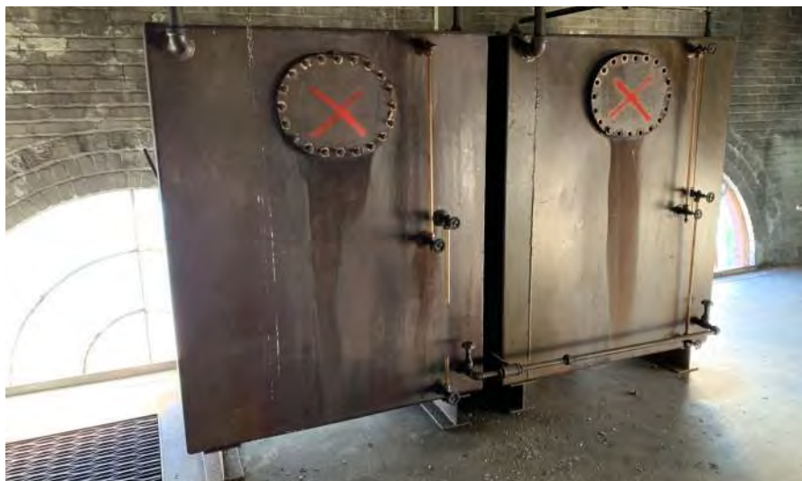
Empty tanks on third floor mezzanine
