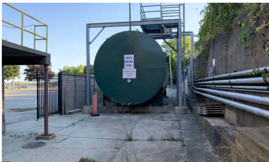
Diesel fuel AST facing northeast
