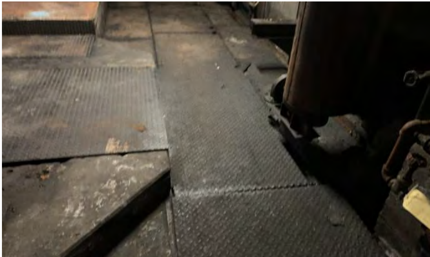
Piping trench covers in basement
