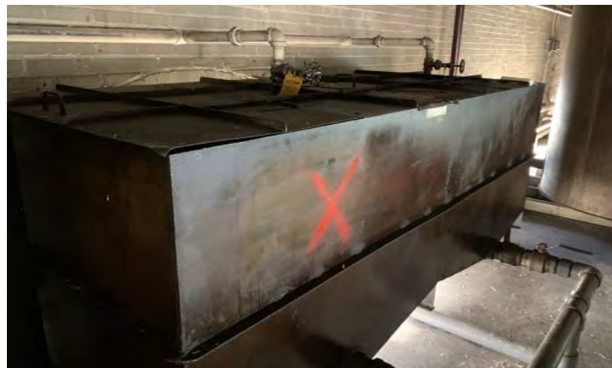
Empty used oil tank on third floor mezzanine
