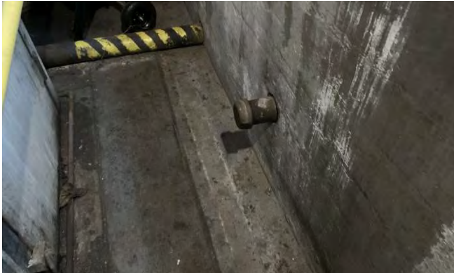
Pipe in basement leading out of north side of building
