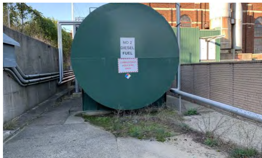
Diesel fuel AST facing southwest
