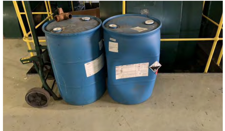
Water treatment chemicals near diesel engine
