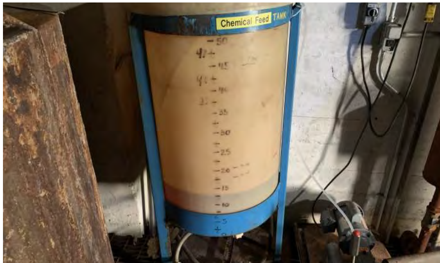
Boiler feed tank in boiler room
