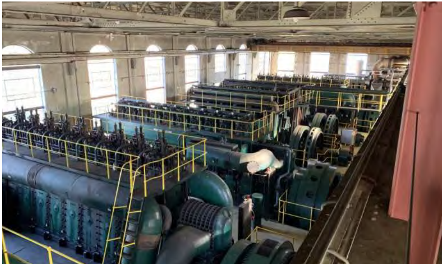
Diesel engines viewed from 3rd floor mezzanine
