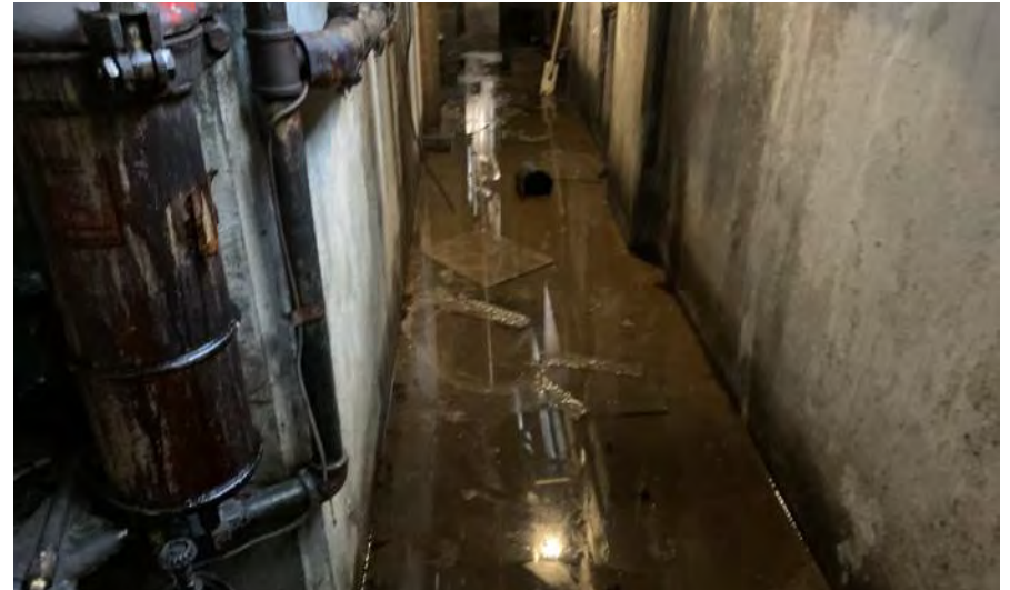
Groundwater accumulation in basement
