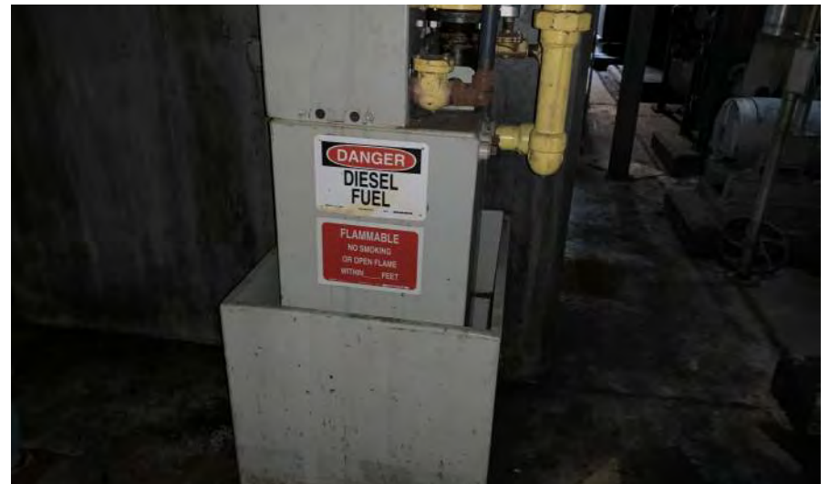
Engine diesel fuel reservoir in basement
