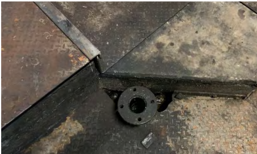
Piping connection in basement
