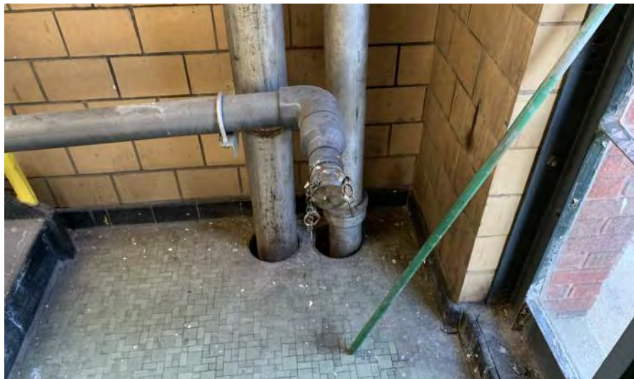
Used oil discharge pipe on second floor mezzanine
