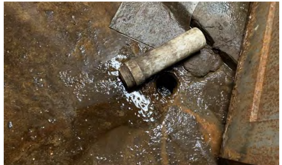
Groundwater in basement flowing into floor drain
