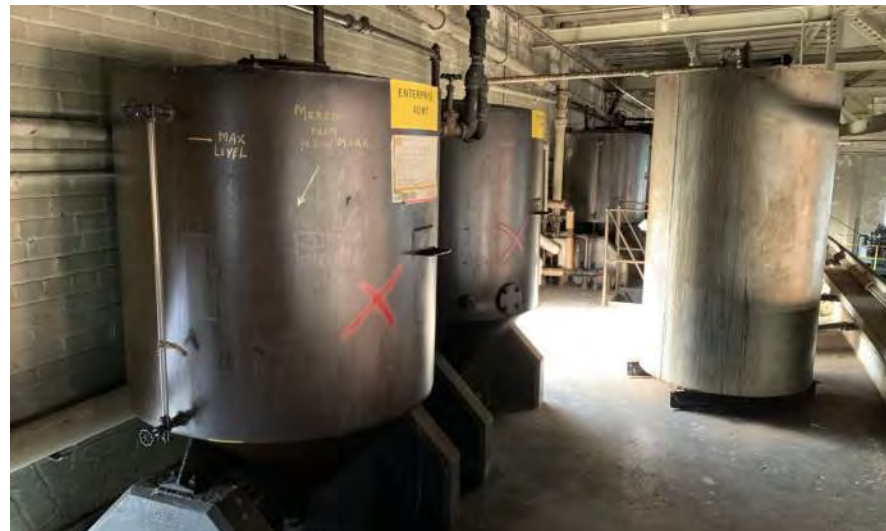
Empty new oil tanks on third floor mezzanine
