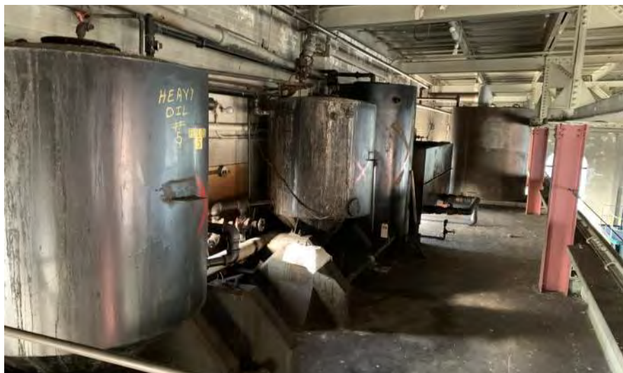
Empty heavy oil and fuel oil tanks on third floor mezzanine
