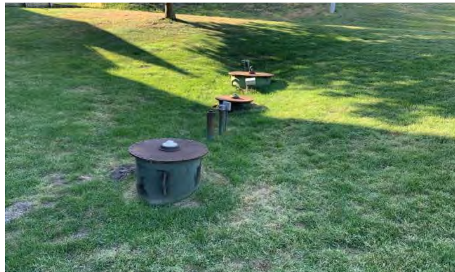
Oil/water separators west of building
