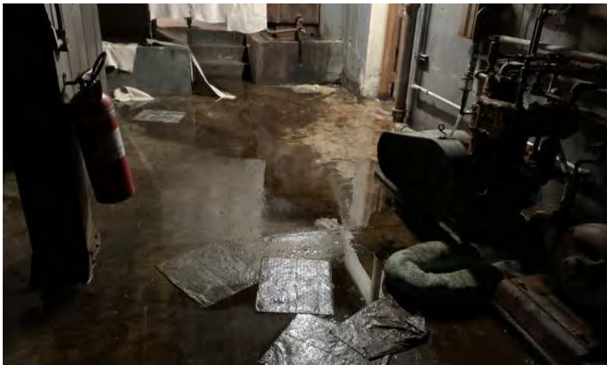
Groundwater accumulation in basement
