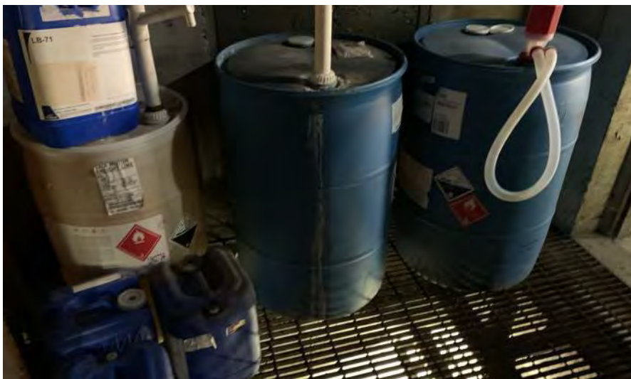
Water treatment chemicals in boiler room
